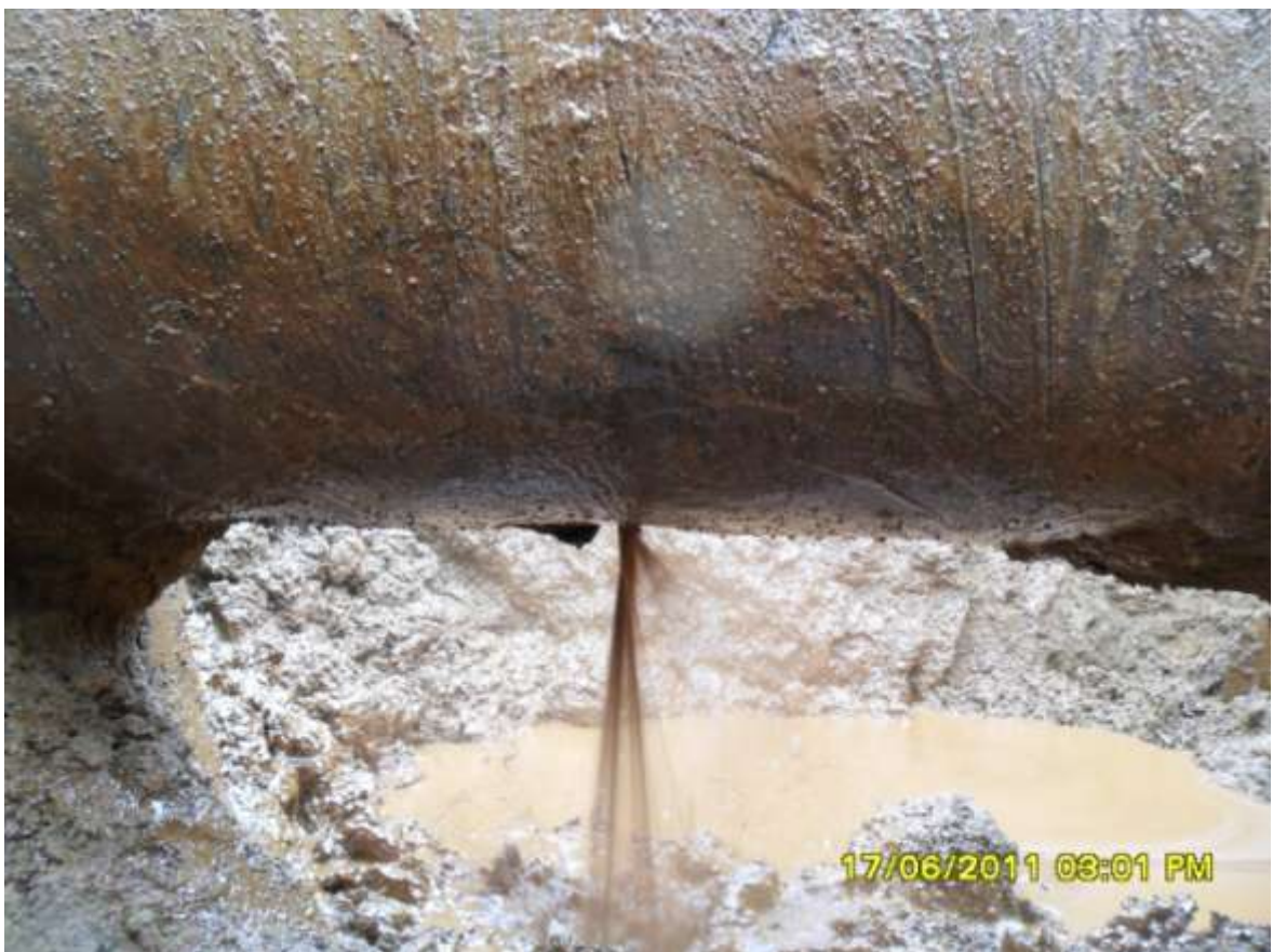
Close-up: Spill due to corrosion between 6 and 7 o'clock position on 24" Nkpoku-Boma pipeline at Akpajo. Picture taken during Joint Investigation of 17 th June, 2011
