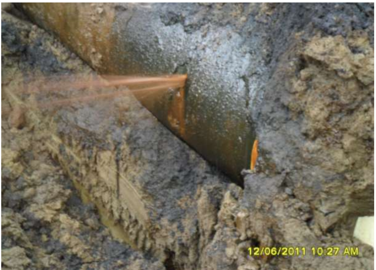
Close-up: Spill due to cut on 24" Bomu-Nkpoku Pipeline at Biara (Ogoni). Picture taken during Joint Investigation of 12 th June, 2011.
