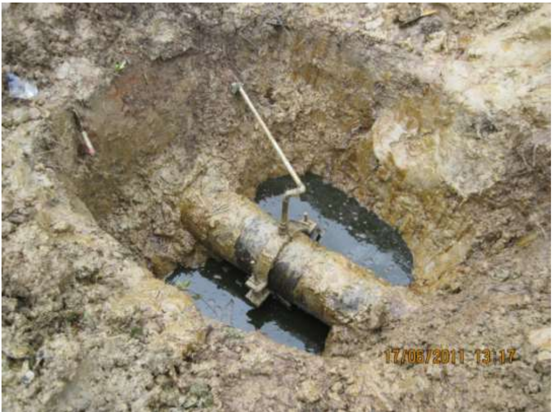
Close-up: Illegally welded fitting on 12" ImoRiver2 pipeline at Odagwa. Picture taken during Joint Investigation of 17 th June, 2011
