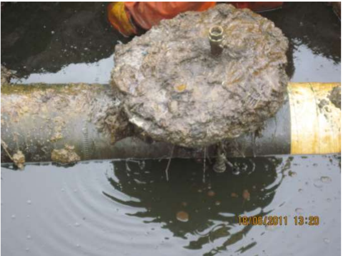
Close-up: Illegally welded fitting on 12" ImoRiver2 pipeline at Odagwa. Picture taken during Joint Investigation of 18 th June, 2011
