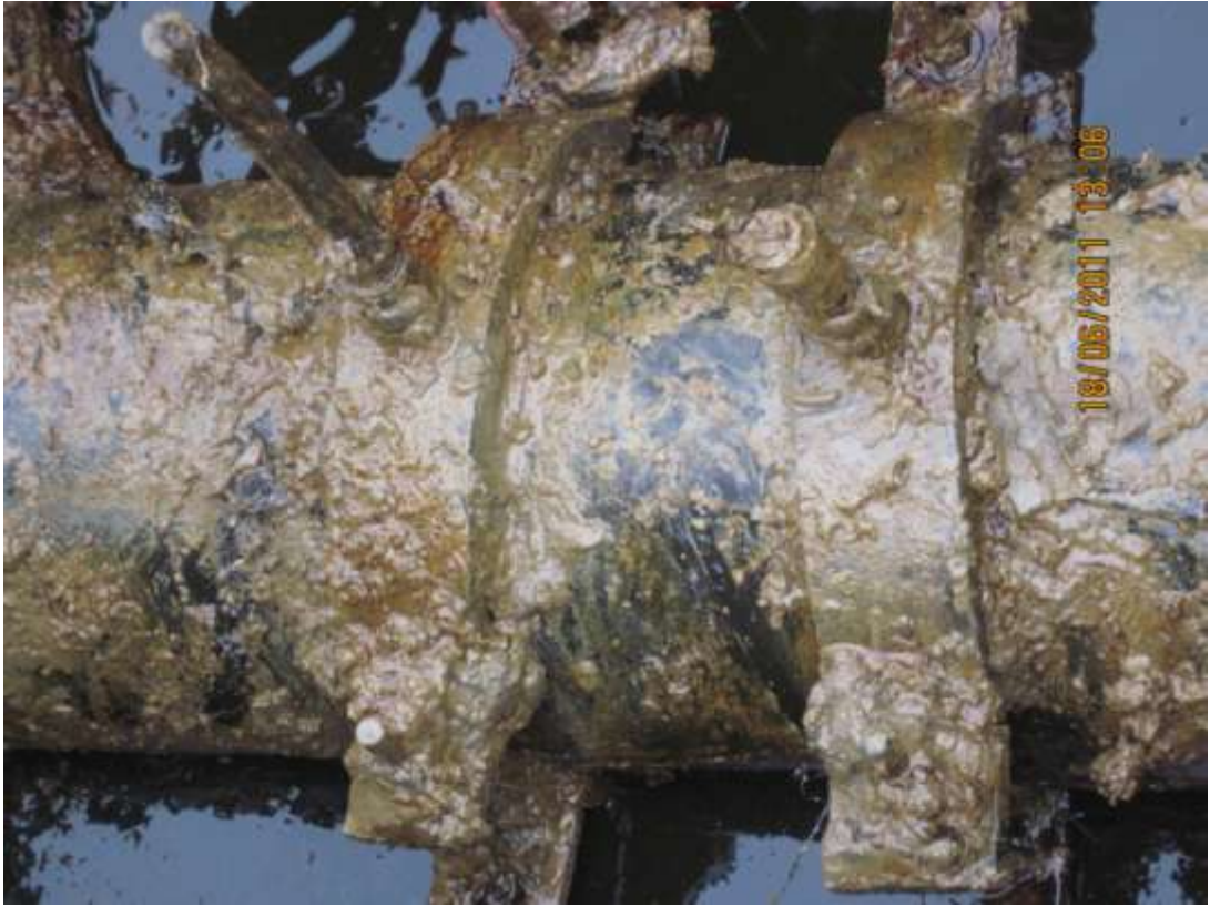
Close-up: Illegally welded fittings on 12" ImoRiver2 pipeline at Odagwa. Picture taken during Joint Investigation of 18 th June, 2011
