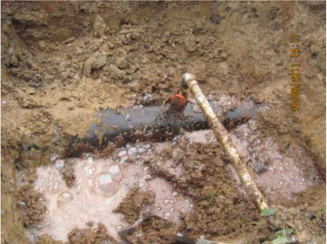
Close-up: Illegally welded fitting on 12" ImoRiver2 pipeline at Odagwa. Picture taken during Joint Investigation of 18 th June, 2011
