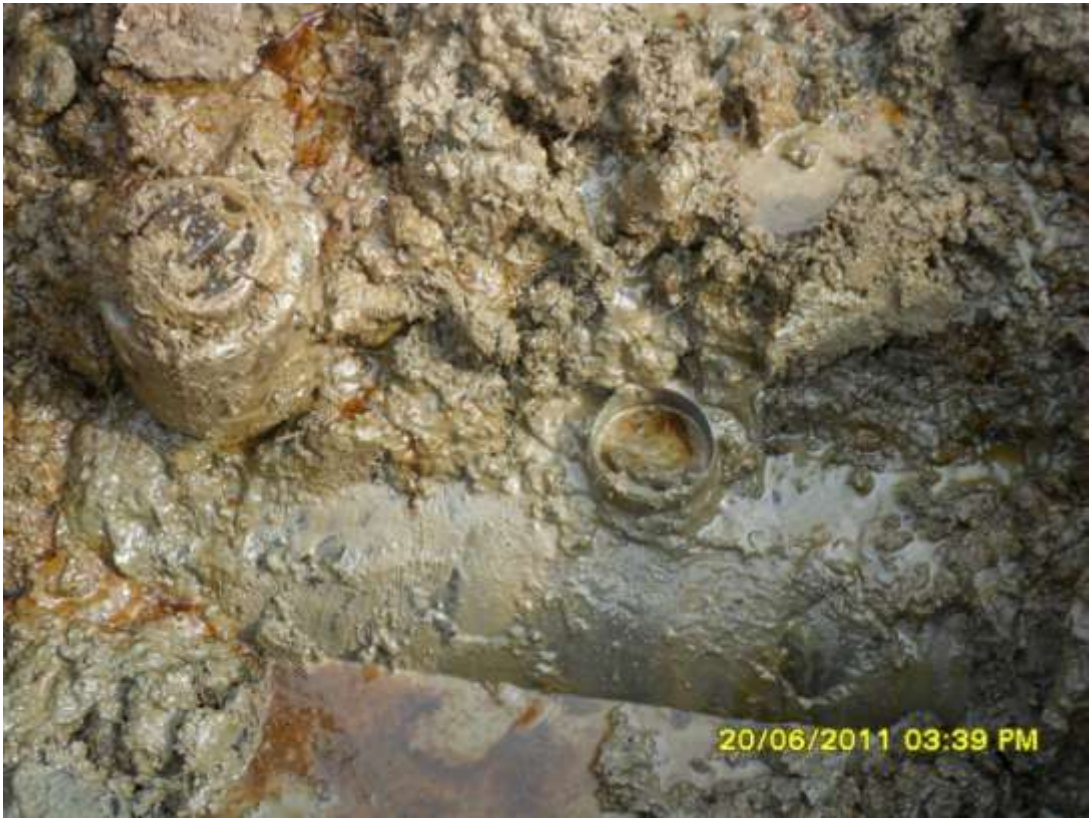
Close-up: Illegal fittings on Okordia-Rumuekpe pipeline and Akalamini riser at Akalamini. Picture taken during Joint Investigation of 20 th June, 2011
