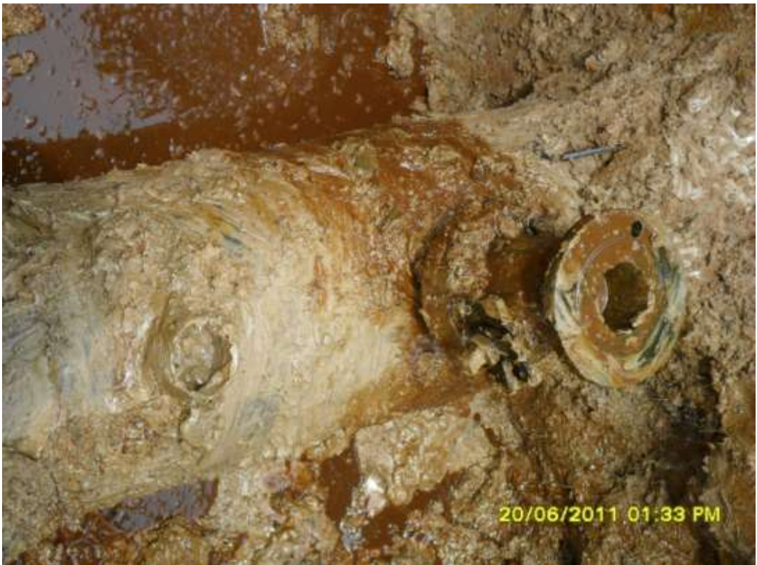
Close-up: Illegal fittings on Okordia-Rumuekpe pipeline and Akalamini riser at Akalamini. Picture taken during Joint Investigation of 20 th June, 2011
