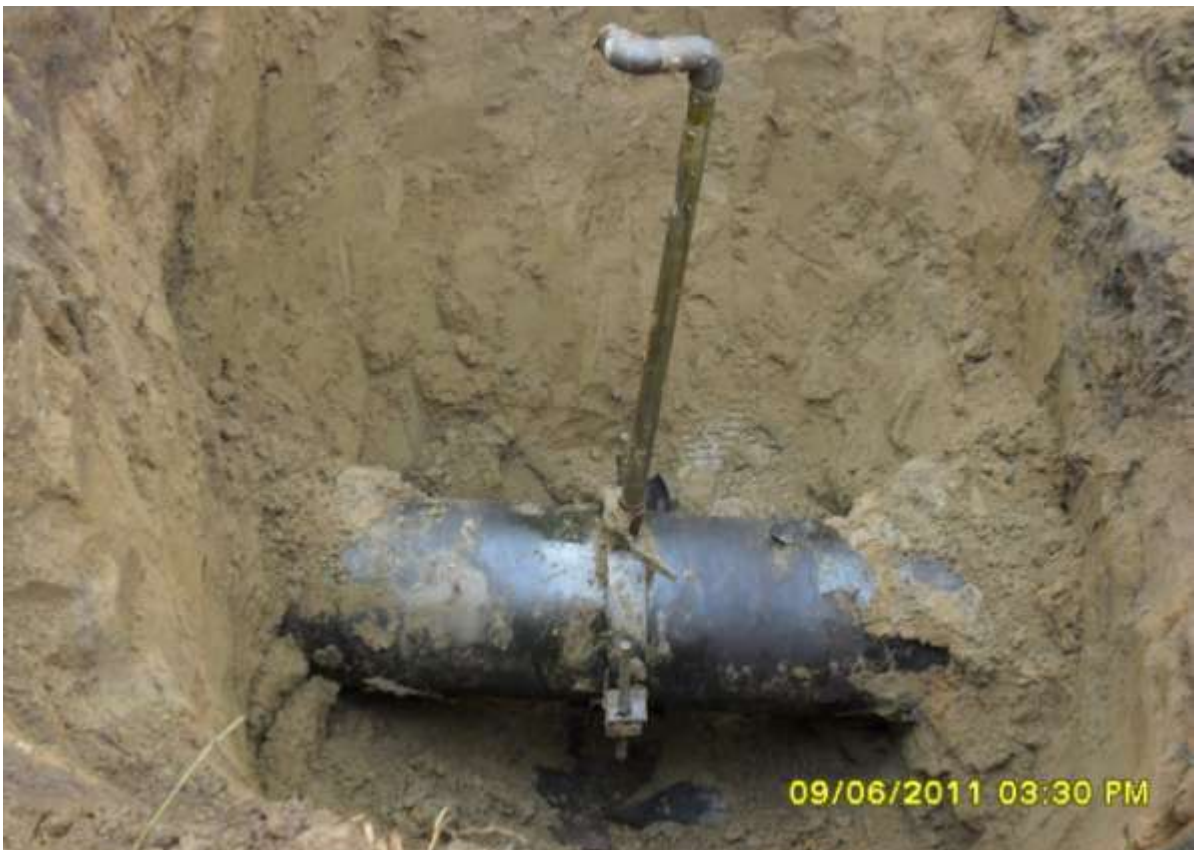
Close-up: Illegally welded fitting on 12" Imo River 1 pipeline in Owaza. Picture taken during Joint Investigation of 9 th June, 2011.
