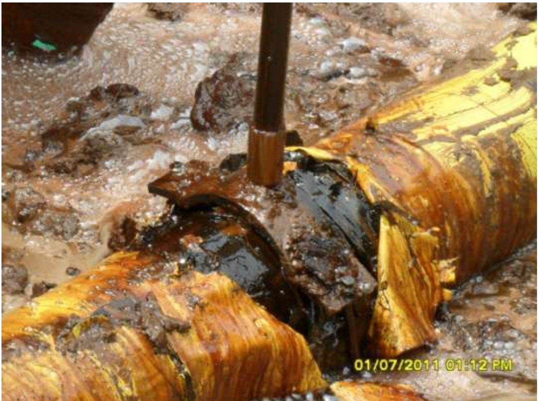
Close-up: Illegal fitting on 8" Isimiri pipeline right of way at Umuaghala. Picture taken during Joint Investigation of 1 st July, 2011
