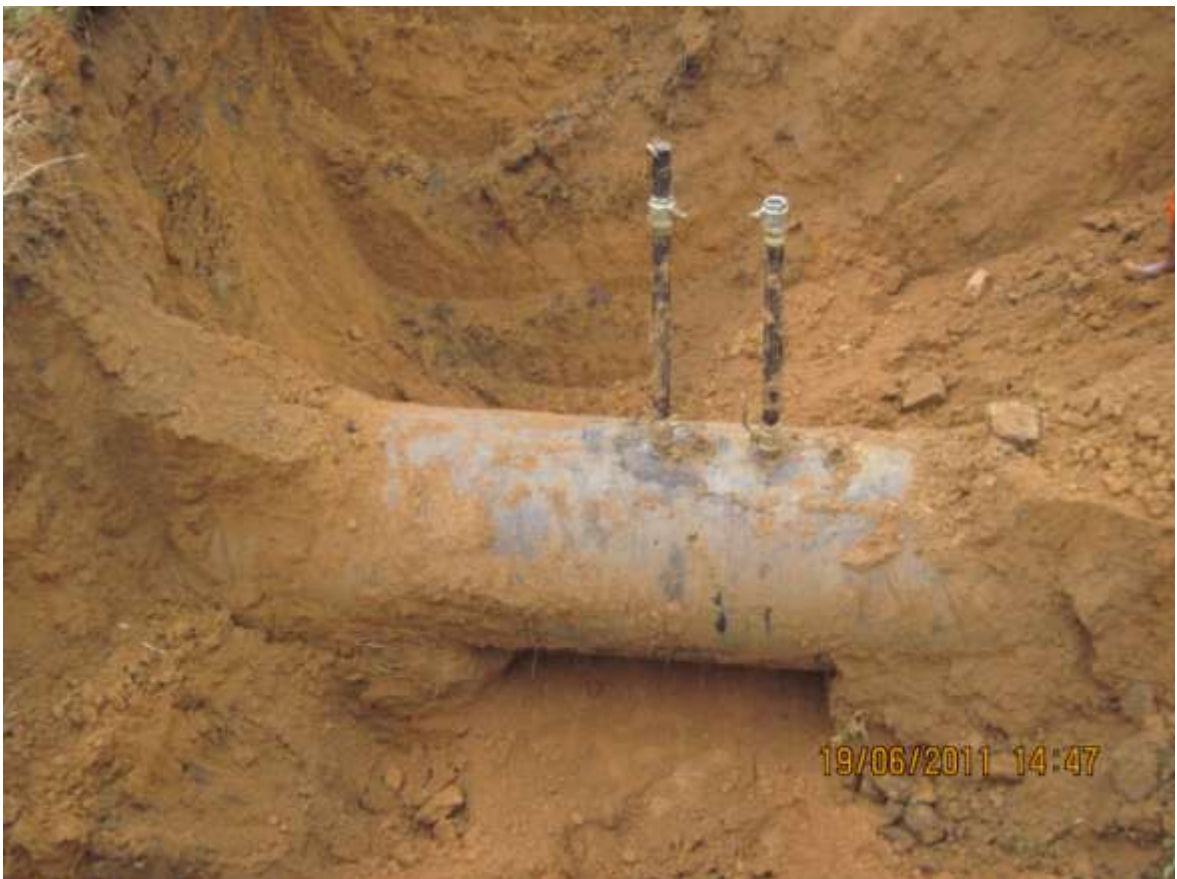
Close-up: Illegally welded fittings on 36" Rumuekpe-Nkpoku pipeline at Aluu. Picture taken during Joint Investigation of 19 th June, 2011
