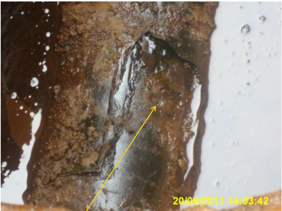
Close-up: Spill from pinhole due to corrosion on 6" bulkline to Agbada2 flowstation at Agbada. Picture taken during Joint Investigation of 20 th June, 2011
