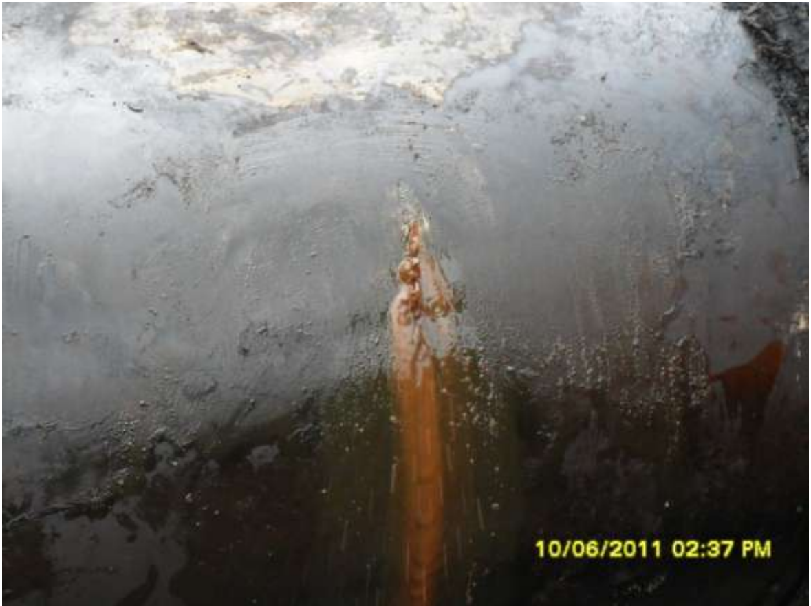
Close-up: Spill due to cut on 24" Bomu- Bonny Pipeline at Bodo (Ogoni). Picture taken during Joint Investigation of 10 th June, 2011.
