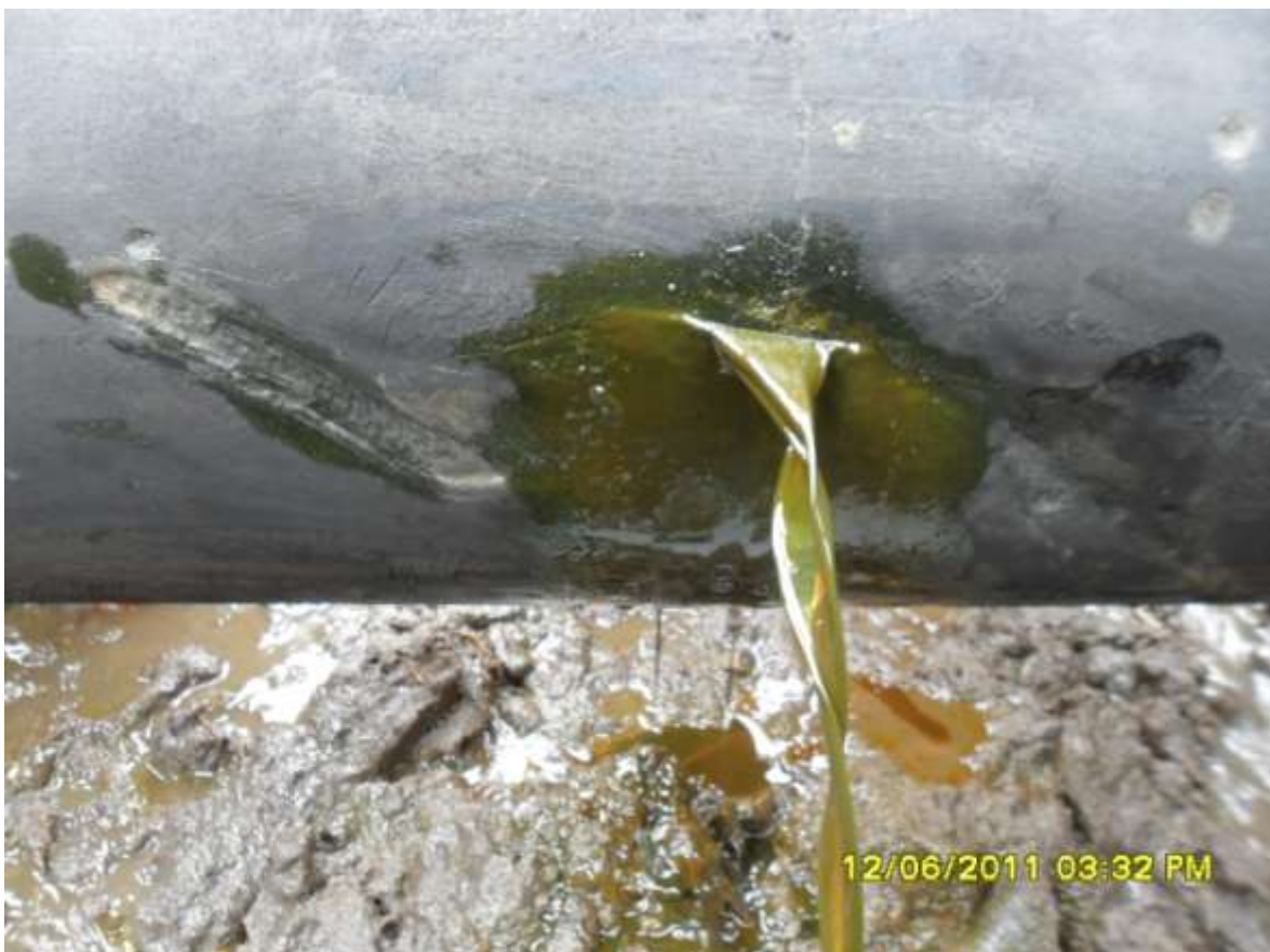
Close-up: Spill due to tear on 10" Ekulama2 delivery line at Ekulama. Picture taken during Joint Investigation of 12 th June, 2011
