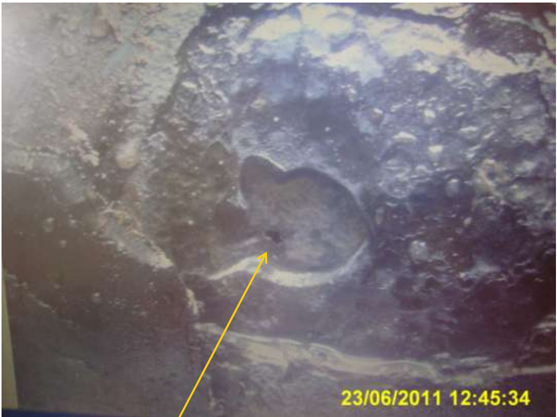
Close-up: Spill point due to corrosion on Cawthorne channel Well 45T flowline at Mbiama. Picture taken during Joint Investigation of 23 rd June, 2011
