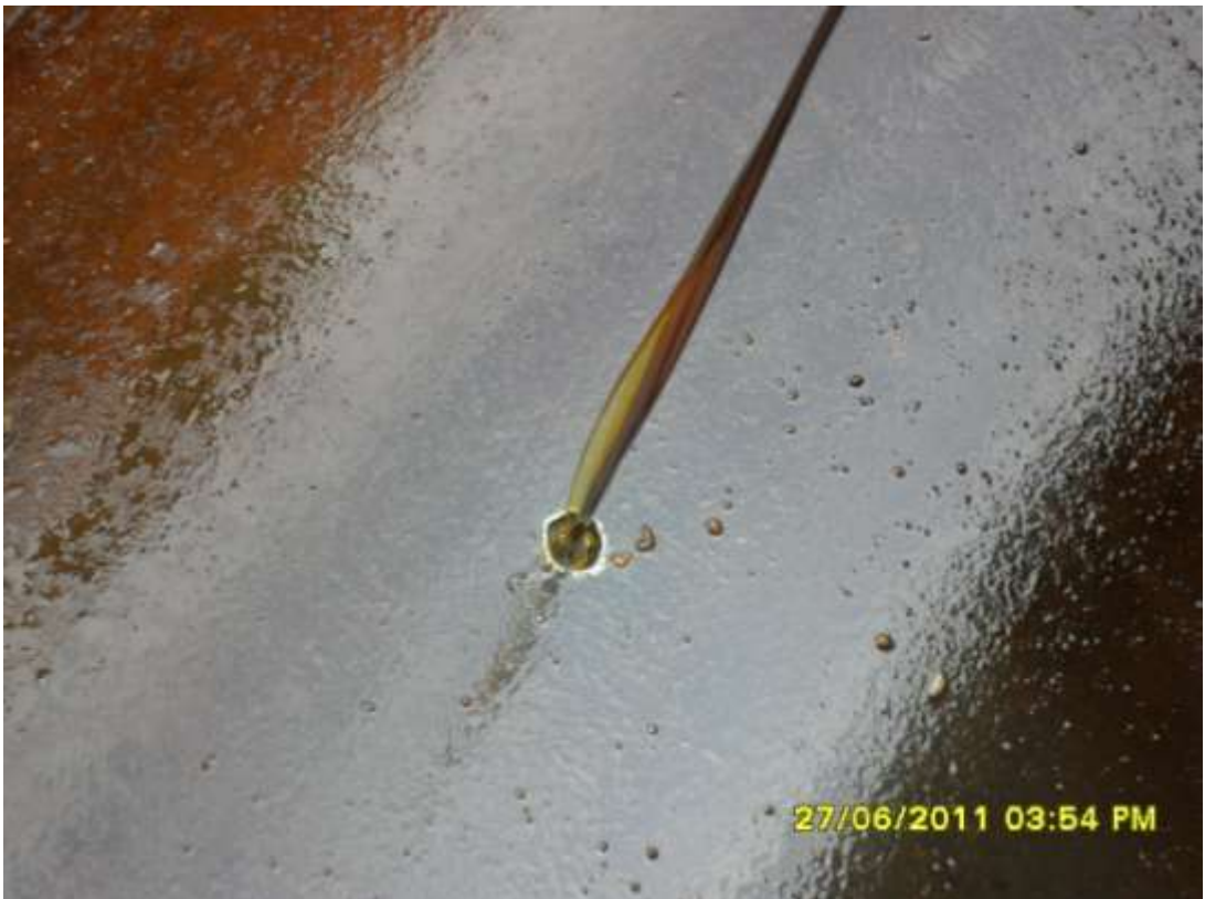
Close-up: Drilled hole on 18" Assa-Rumuekpe pipeline at Awara. Picture taken during Joint Investigation of 27 th June, 2011
