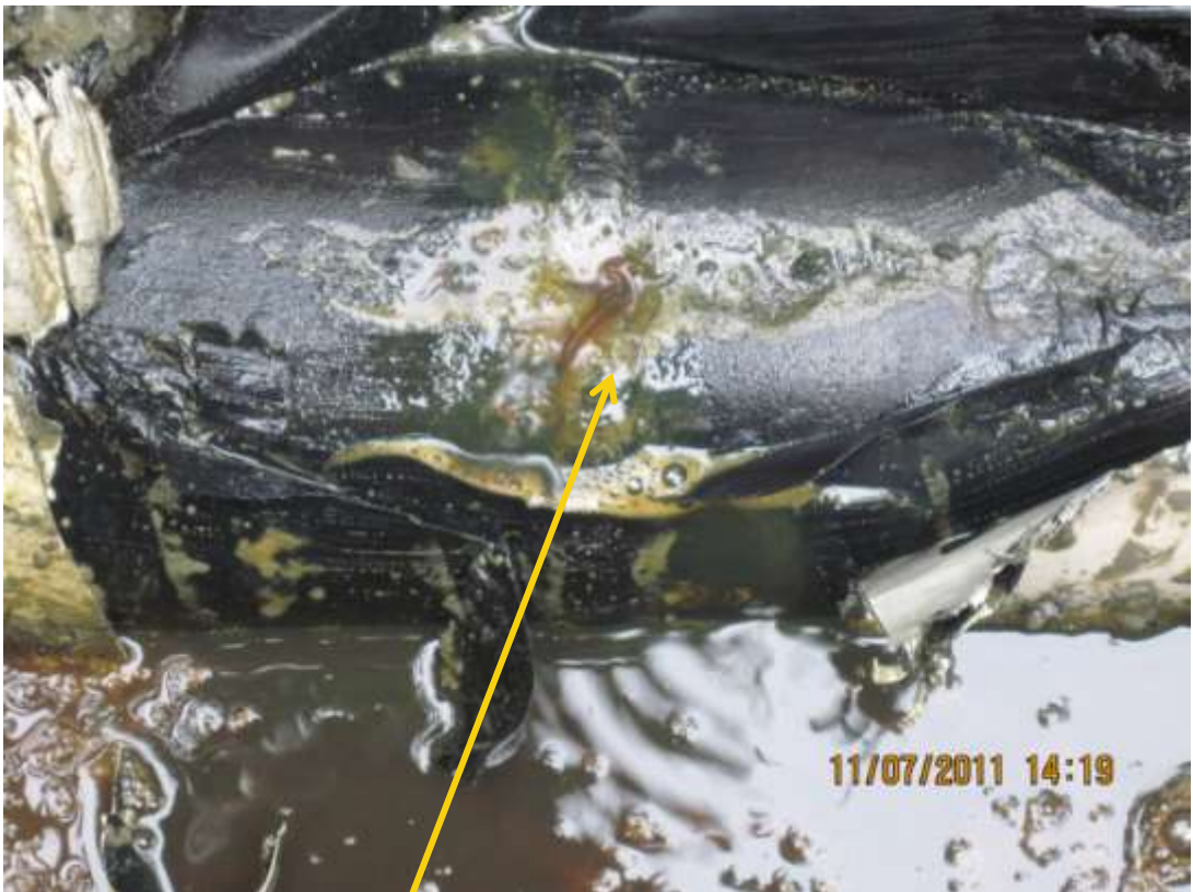
Close-up: Spill due to drilled hole on Nun River Well15S flowline at Onyoma. Picture taken during Joint Investigation of 11 th July, 2011
