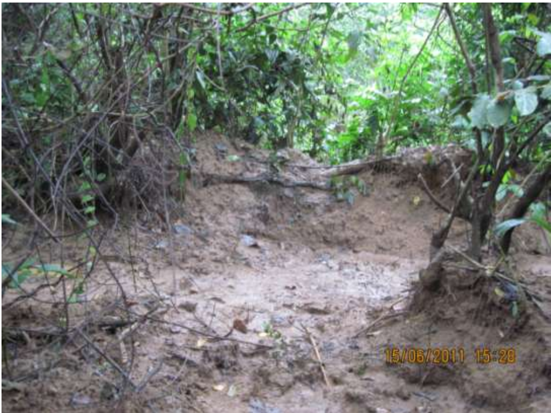
Overview: Spill point area after repair on Imo River Well59T flowline Right of Way at Igiukwu. Picture taken during Joint Investigation of 15 th June, 2011
