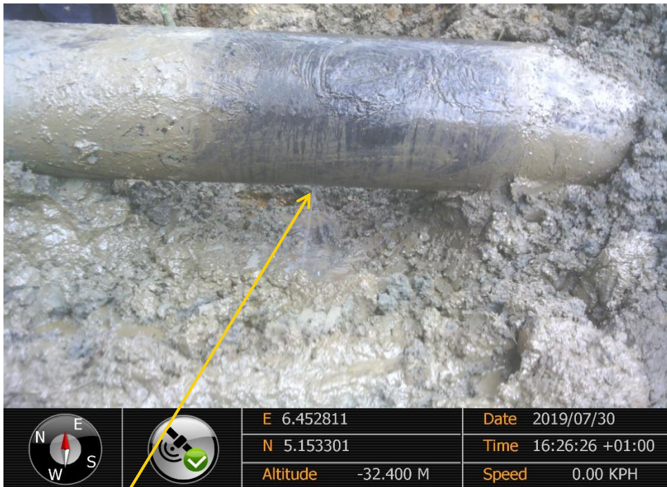
Close-up: Internal Corrosion on 14" Okordia - Rumuekpe Pipeline at Ikarama. Picture was taken during Joint Investigation of 30 th July 2019
