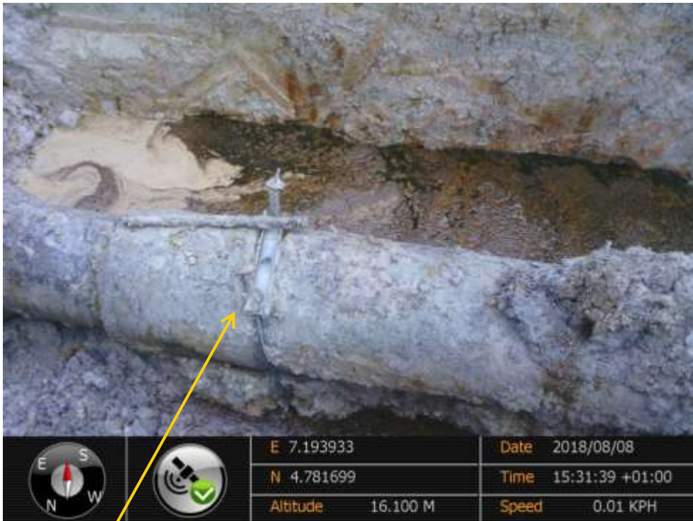
Close-up: Locally fabricated clamp on 24" Nkpoku-Bomu Pipeline at Sime. Picture was taken during Joint Investigation of 8 th August 2018.
