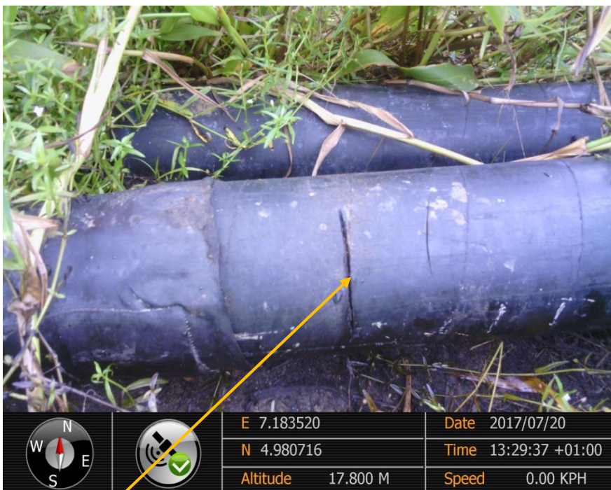
Close-up: Hacksaw Cut on Imo River 3 Well 22S Flowline at Igiriukwu-Owaza. Picture was taken during Joint Investigation of 20 th July 2017.
