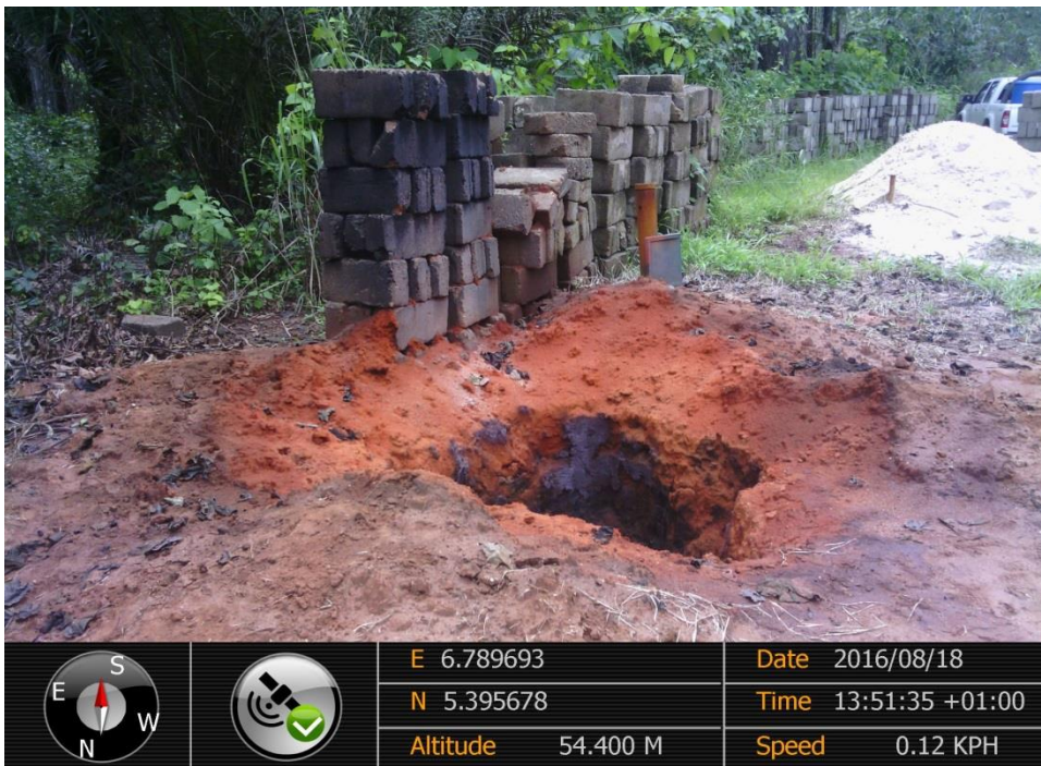
Overview: Part of spill impact on 16" Egbema-Assa Pipeline at Obile. Picture was taken during Joint Investigation of 18 th August 2016.
