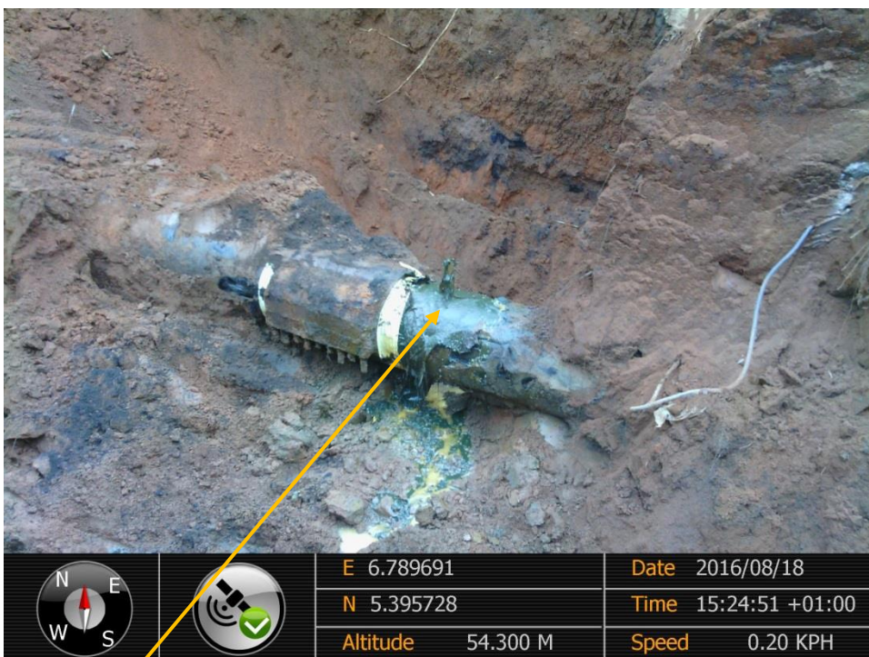
Close-up: Drilled hole on 16" Egbema-Assa Pipeline at Obile. Picture was taken during Joint Investigation of 18 th August 2016.
