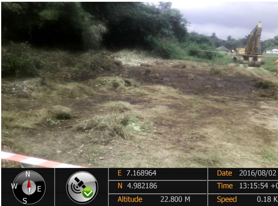
Overview: Part of spill impact on 12" Imo River 2–Ogale Pipeline at Umuedeokwara. Picture was taken during Joint Investigation of 2 nd August 2016.
