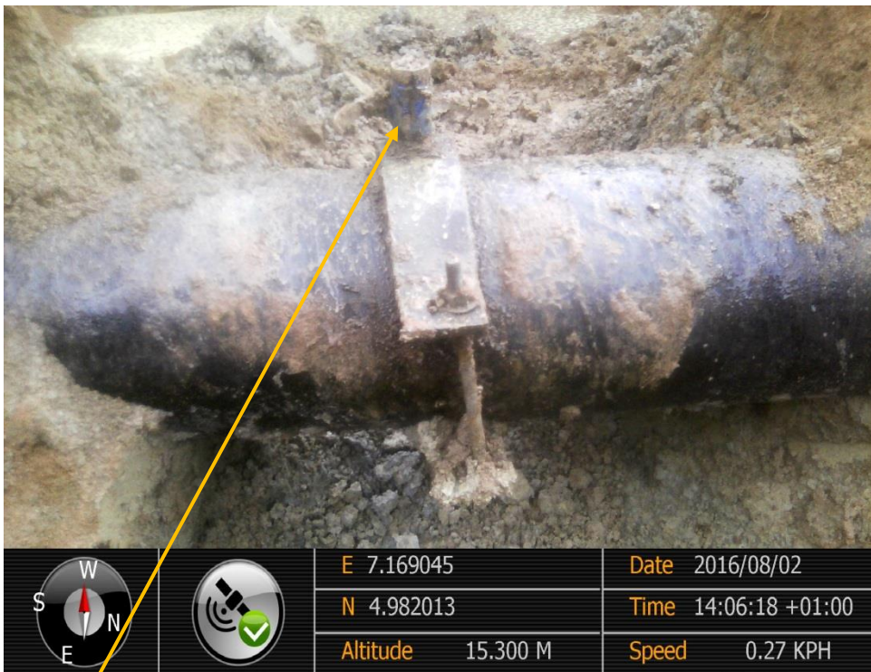
Close-up: Illegal fitting on 12" Imo River 2–Ogale Pipeline at Umuedeokwara. Picture was taken during Joint Investigation of 2 nd August 2016.
