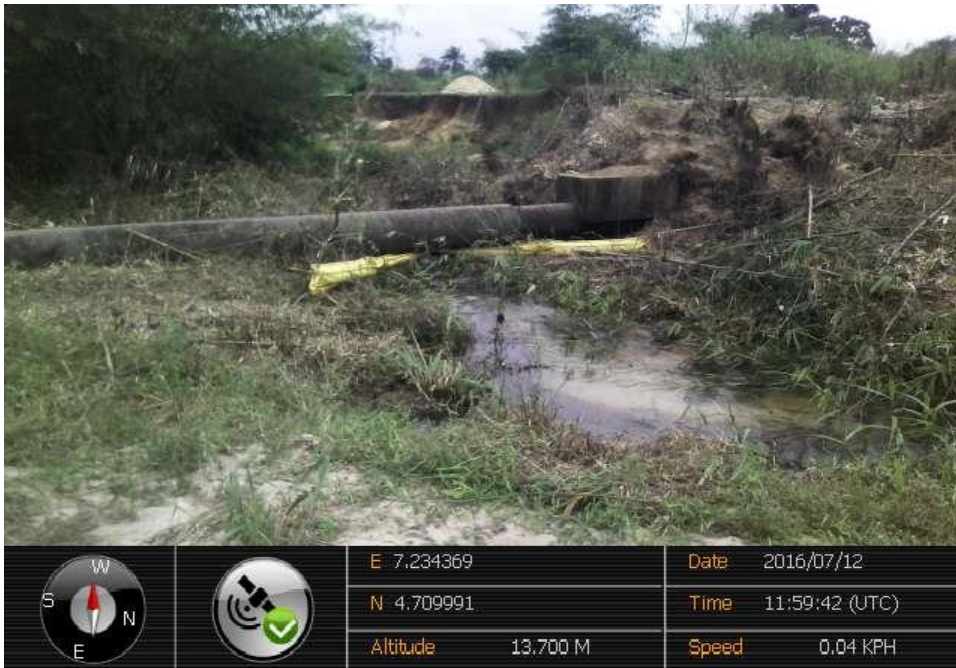
Overview: Part of spill impact on 28" Nkpoku - Bomu Pipeline at Gio – Kporghor. Picture was taken during Joint Investigation of 12 th July 2016.
