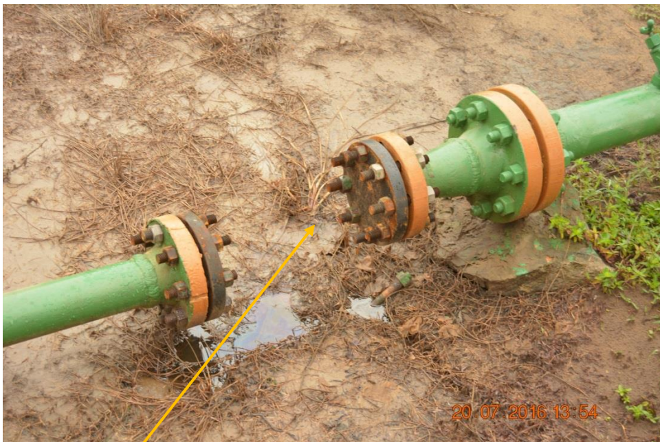
Close-up: Position of stolen 3" plug valve on Yokri Well 113T Flowline at Obotobo I & II. Picture was taken during Joint Investigation of 20 th July 2016.
