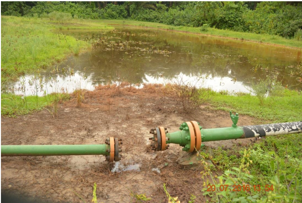
Overview: Part of spill impact on Yokri Well 113T Flowline at Obotobo I & II. Picture was taken during Joint Investigation of 20 th July 2016.
