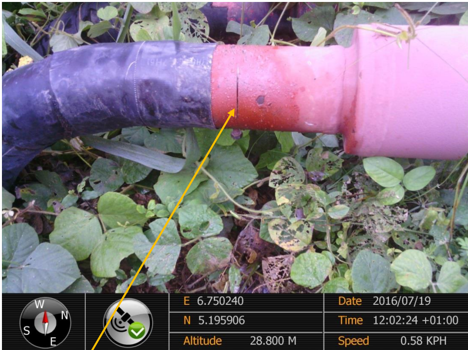
Close-up: Hack Saw Cut on Ahia Well 3S Flowline at Egbeda. Picture was taken during Joint Investigation of 19 th July 2016.
