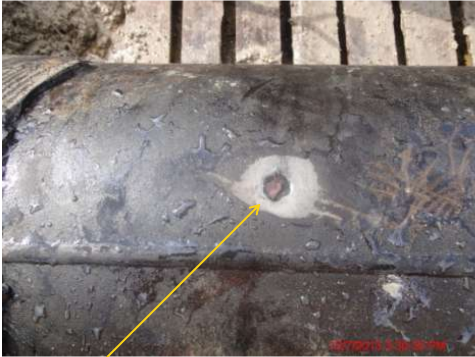
Close up : Drilled hole plugged with a wooden peg on 20" Rumuekpe-Nkpoku pipeline at Ibaa. Picture was taken during Joint Investigation of 12 th July 2013.
