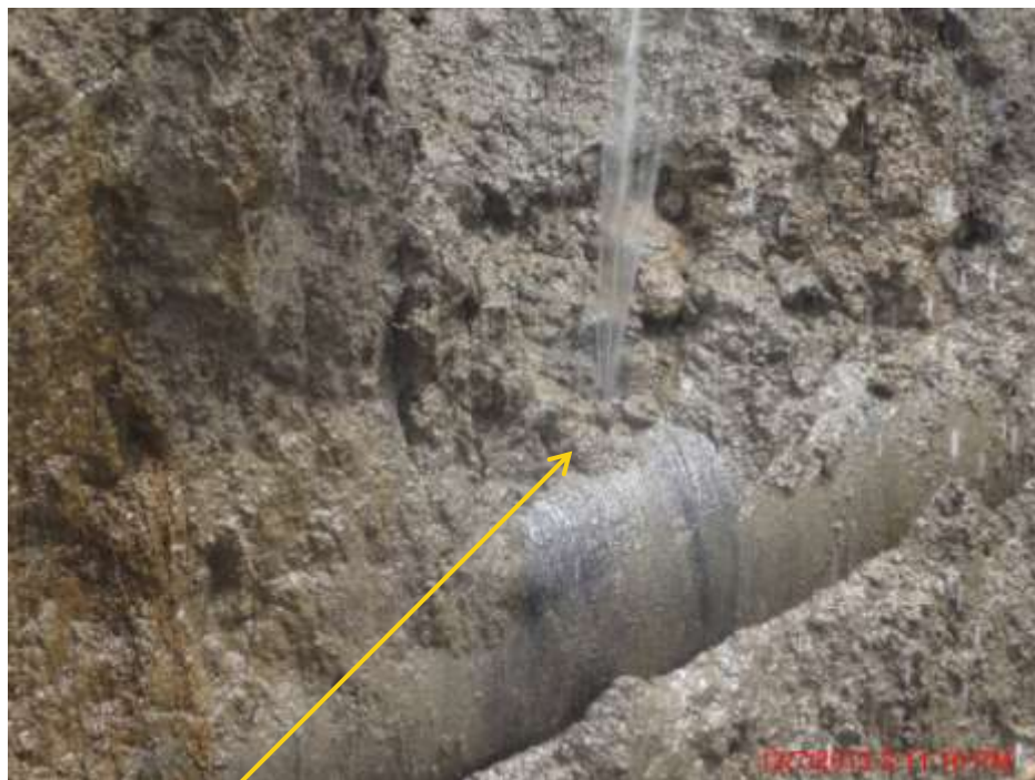
Close up: Drilled hole before plugging on 20" Rumuekpe-Nkpoku pipeline at Ibaa. Picture was taken during Joint Investigation of 12 th July 2013.
