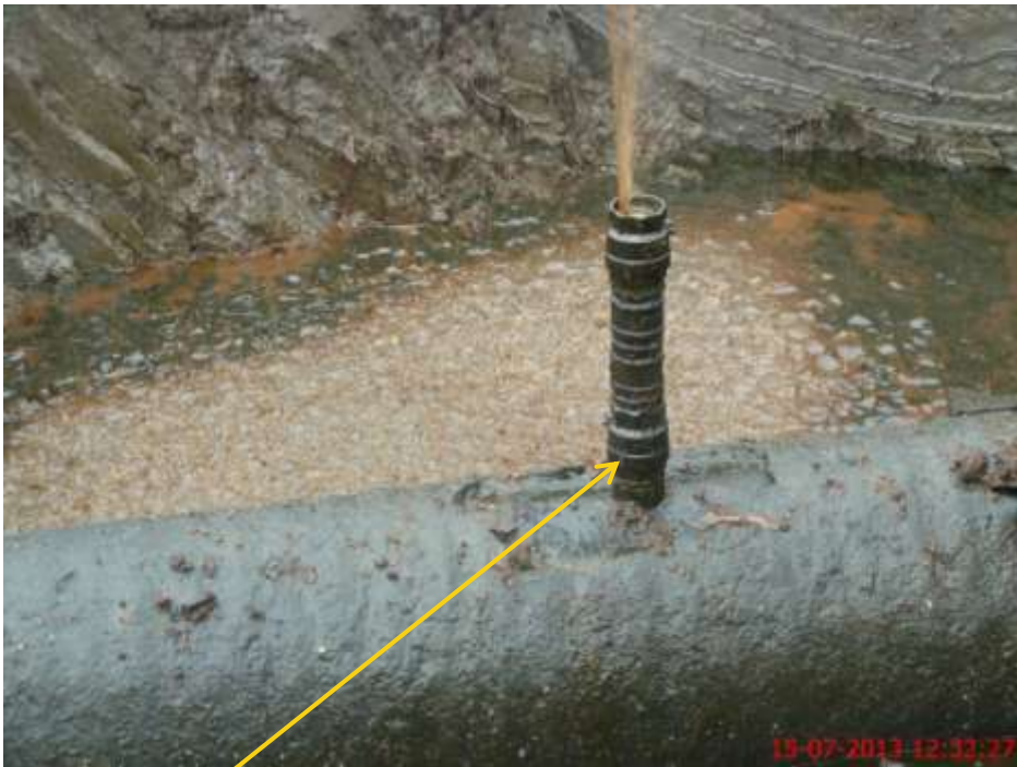
Close up: Illegal fitting on 24" Bomu-Bonny Trans Niger pipeline at Bodo West. Picture was taken during Joint Investigation of 15 th July 2013.
