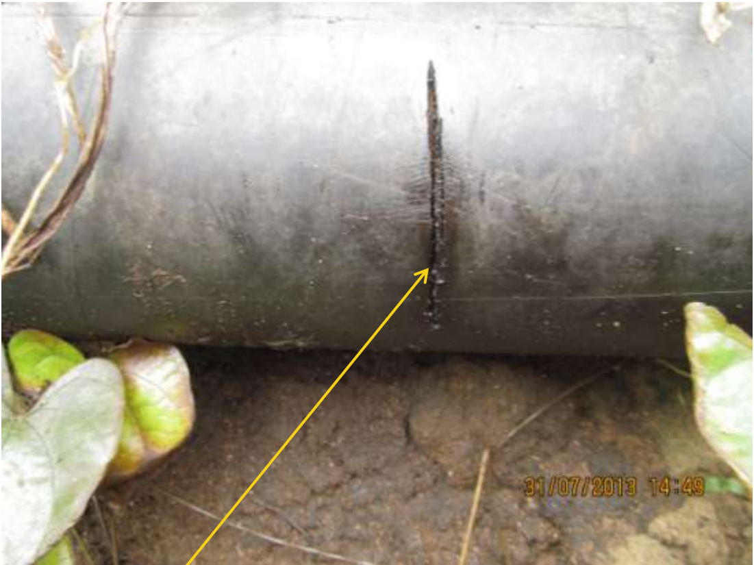
Close up: Hacksaw cut on 4" Imo River Well55S flowline at Igiriukwu. Picture was taken during Joint Investigation of 31 st July 2013.
