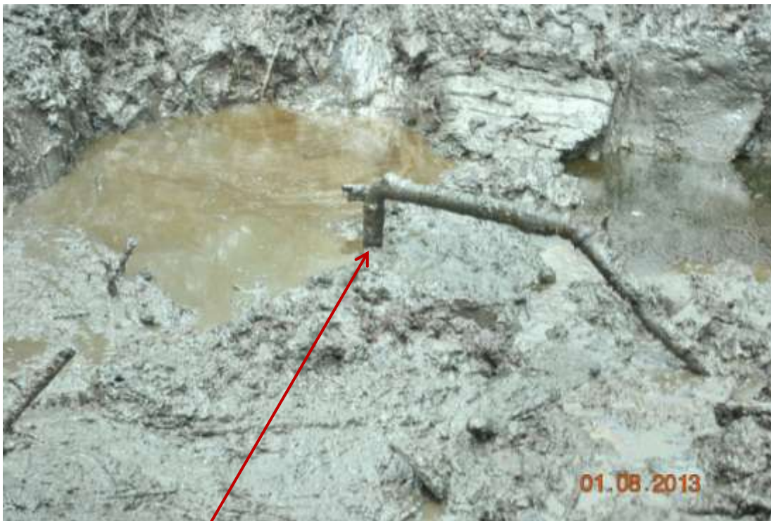
Close up: Illegal fitting on 20" Otumara-Escravos pipeline at Ugboegungun. Picture was taken during Joint Investigation of 1 st August 2013.
