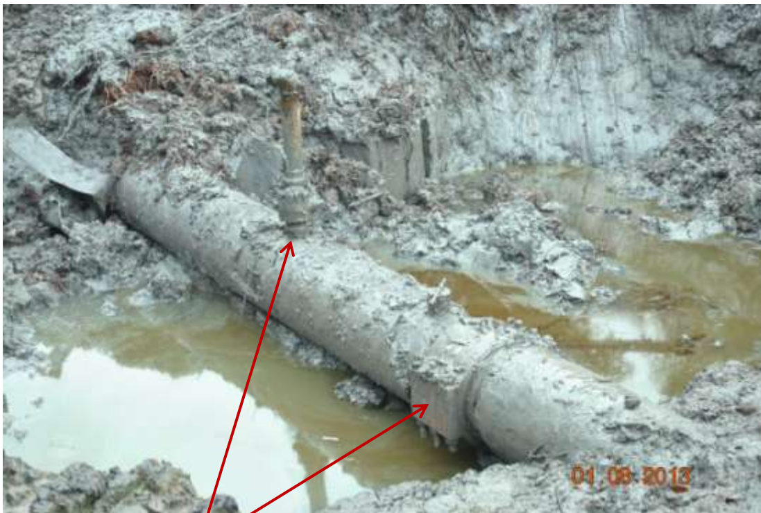
Close up: Illegal fittings on 20" Otumara-Escravos pipeline at Ugboegungun. Picture was taken during Joint Investigation of 1 st August 2013.
