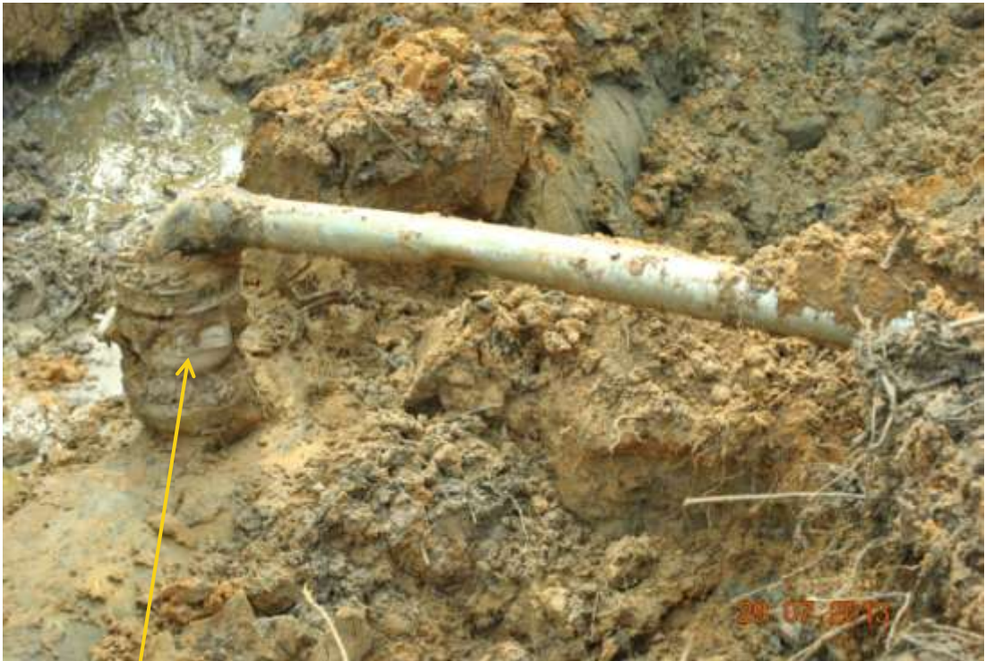
Close up: Illegal fitting on 20" Otumara-Escravos pipeline at Ugboegungun. Picture was taken during Joint Investigation of 29 th August 2013.
