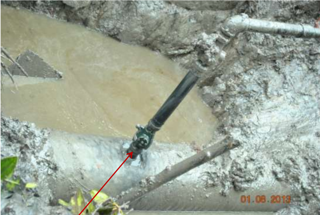
Close up: Illegal fitting on 20" Otumara-Escravos pipeline at Ugboegungun. Picture was taken during Joint Investigation of 1 st August 2013.
