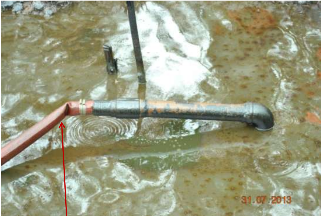
Close up: Illegal fitting on 20" Otumara-Escravos pipeline at Ugboegungun. Picture was taken during Joint Investigation of 31 st July 2013.
