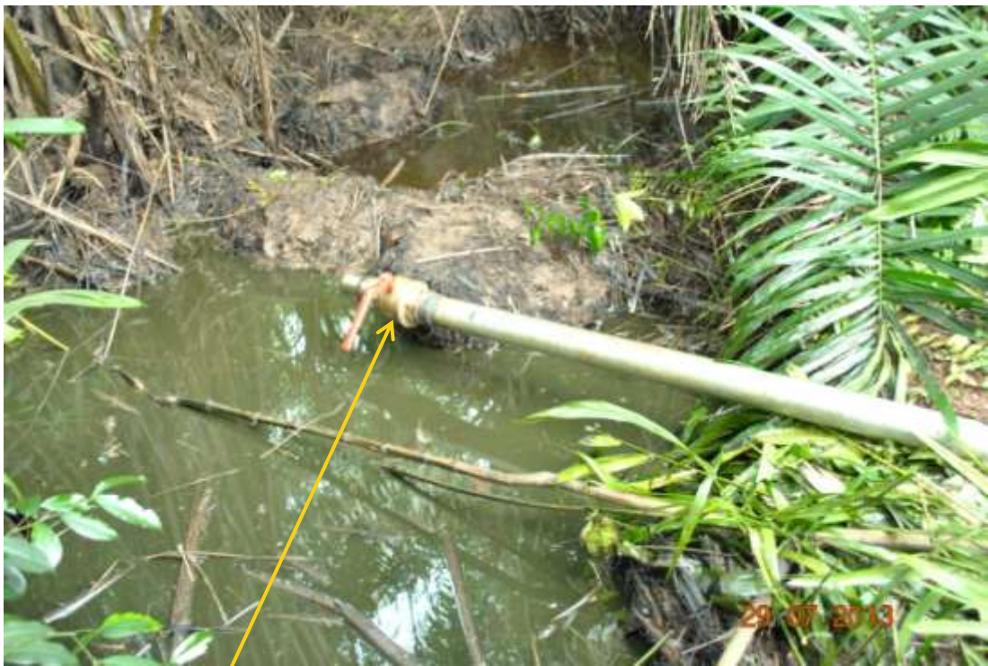
Close up: Illegal fitting on 20" Otumara-Escravos pipeline at Ugboegungun. Picture was taken during Joint Investigation of 29 th August 2013.
