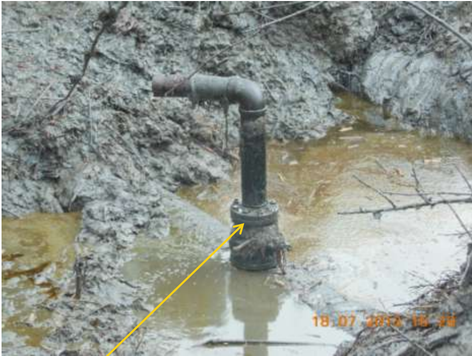
Close up: Illegal fitting on 24" Bomu-Bonny Trans Niger pipeline at Otokomabie/Oloma. Picture was taken during Joint Investigation of 18 th July 2013.
