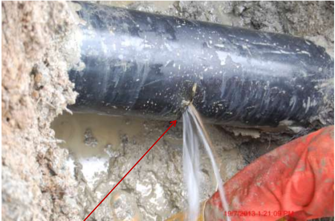
Close up (Point A): Hacksaw cut on 12" Adibawa-Okordia pipeline at Ikarama. Picture was taken during Joint Investigation of 19 th July 2013.
