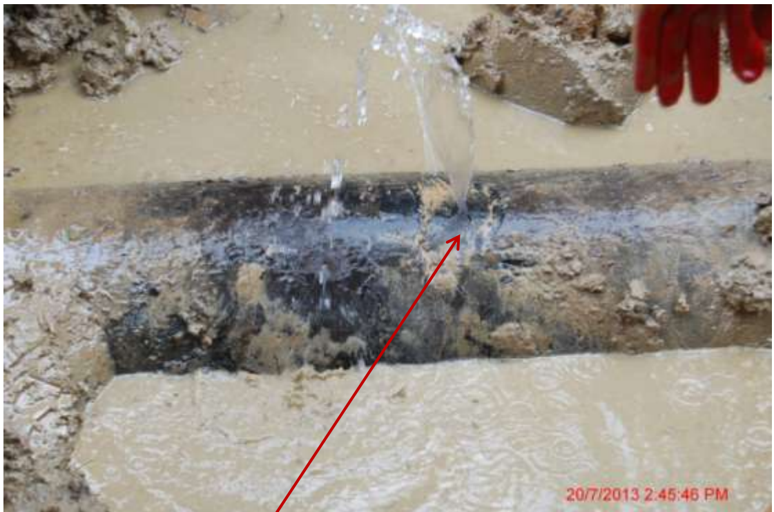
Close up (Point B) : Hacksaw cut on 12" Adibawa-Okordia pipeline at Ikarama. Picture was taken during Joint Investigation of 20 th July 2013.
