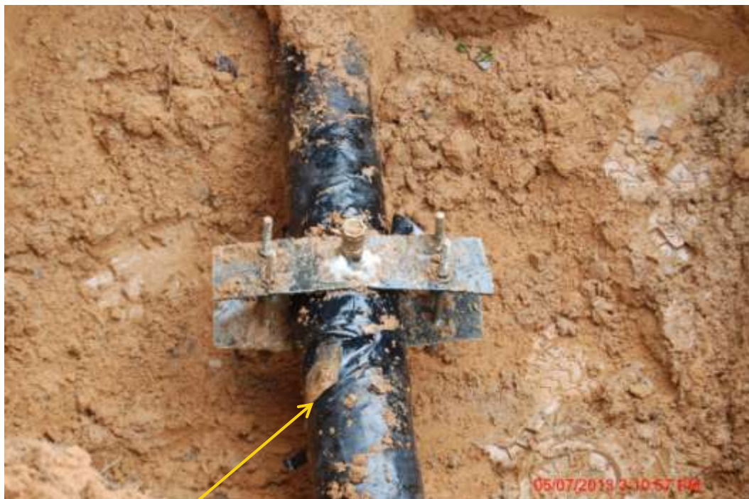
Close up: Illegal fitting on 6" Obigbo North – Ogale pipeline at Ogale. Picture was taken during Joint Investigation of 5 th July 2013.
