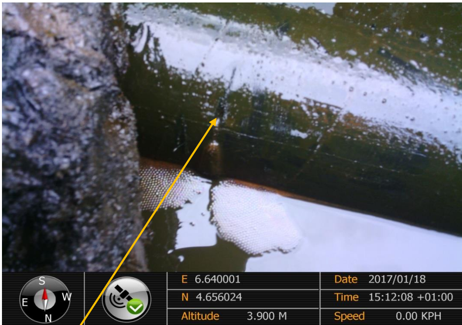
Close-up: Hacksaw cut on Soku Well 21L Flowline at Russia-Soku. Picture was taken during Joint Investigation of 18 th January 2017.
