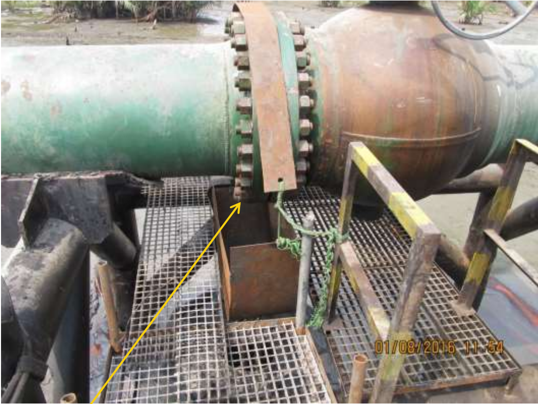
Close-up: Leak point on 28" Bomu-Bonny Pipeline (Opobo Riser) at Owokori. Picture was taken during Joint Investigation of 8 th January 2016.
