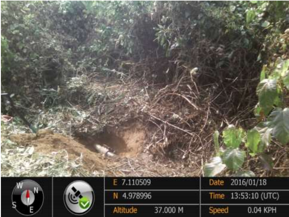
Overview: Part of spill impact on 4" Nkali Well10S Flowline Right of Way at Odagwa2. Picture was taken during Joint Investigation of 18 th January 2016.
