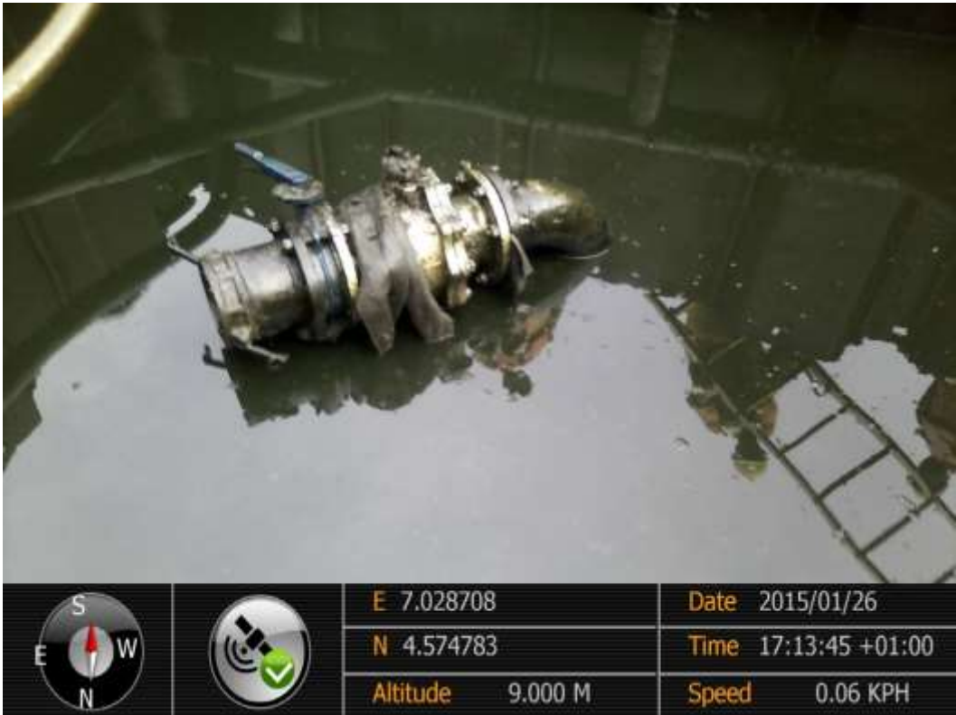
Close-up: Illegal fitting on 30" Nembe Creek Pipeline at Opomakiri. Picture was taken during Joint Investigation of 26 th January 2015.
