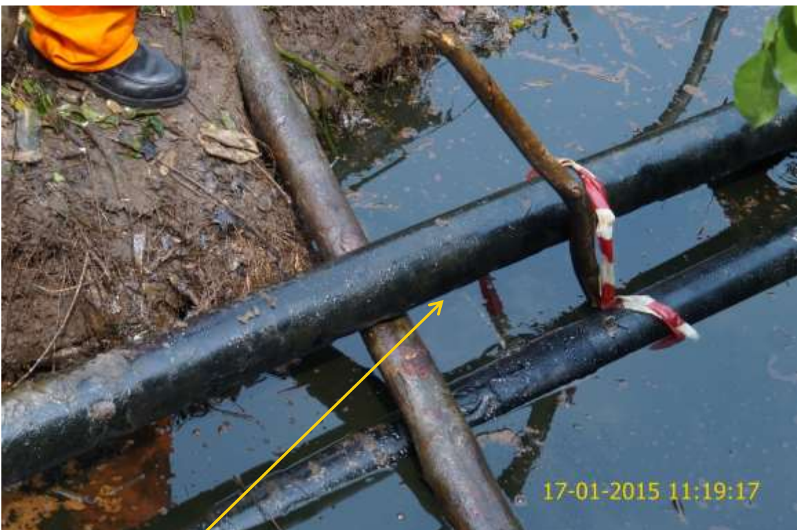
Close-up: Spill due to corrosion on 4" Yokri Well 114L Flowline at Yokri. Picture was taken during Joint Investigation of 17th January 2015.
