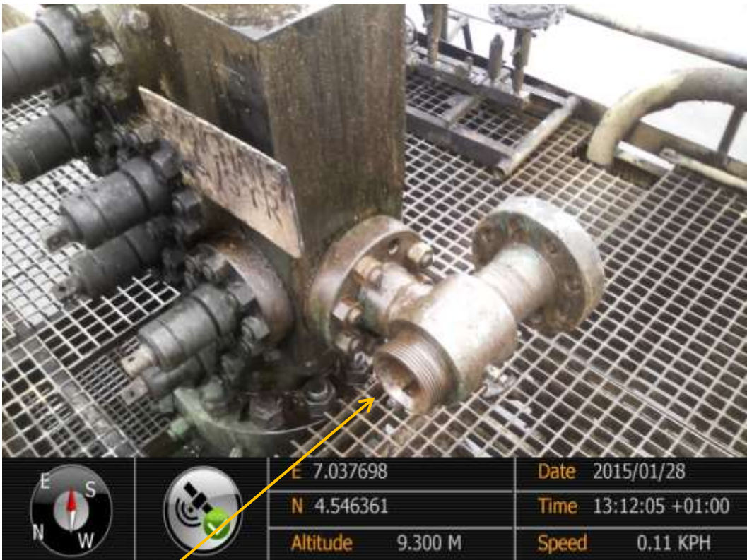
Close-up: Spill point on Cawthorne Channel1 Well9 at Captainkiri. Picture was taken during Joint Investigation of 28 th January 2015.
