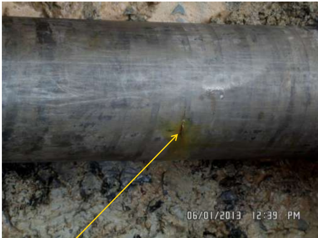
Close up: Hacksaw cut on 10" Diebu Creek – Nun River pipeline at Onyoma. Picture was taken during Joint Investigation of 6 th January 2013.
