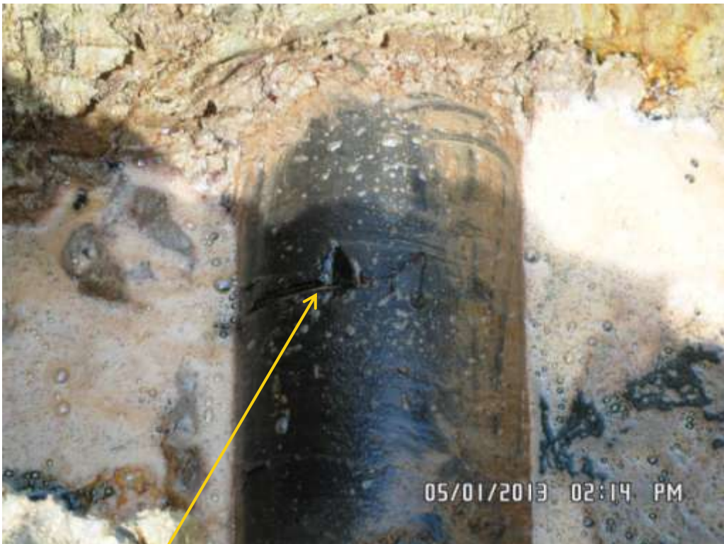
Close up: Hacksaw cut on 10" Diebu Creek – Nun River pipeline at Onyoma. Picture was taken during Joint Investigation of 5 th January 2013.
