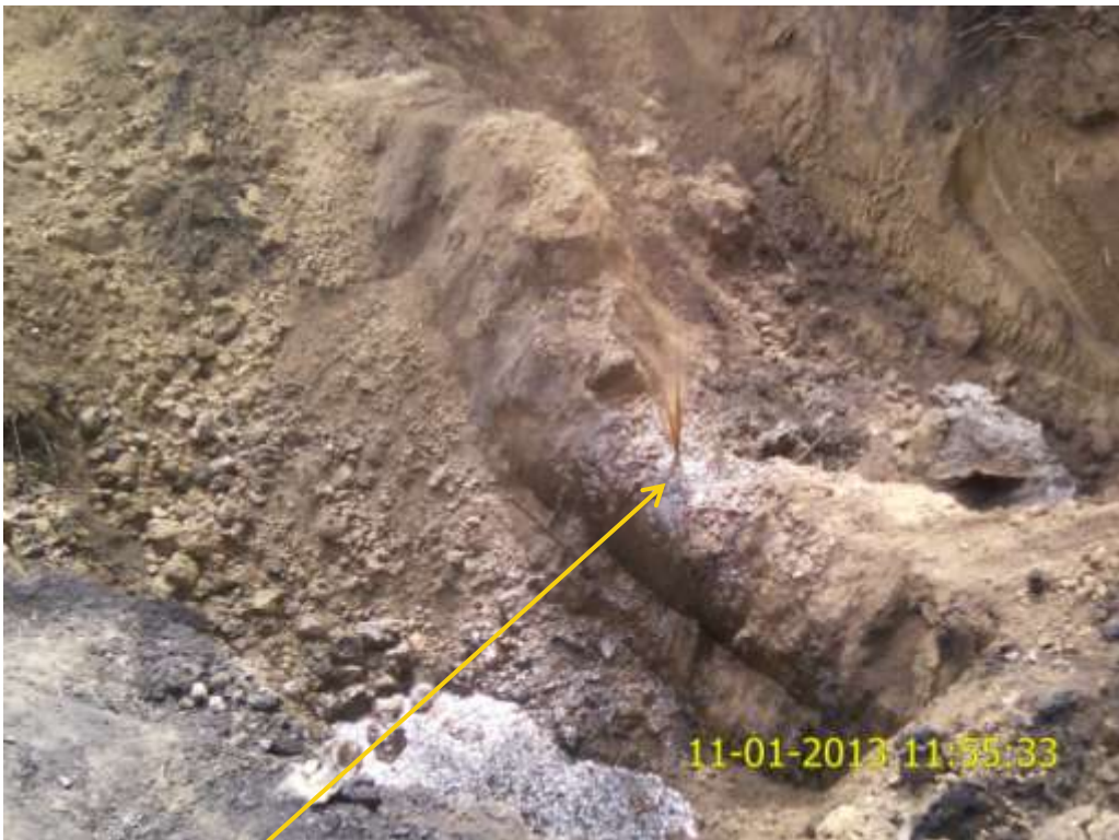
Close up: Spill due to drilled hole on 24" Nkpoku-Bomu pipeline at Sime Picture was taken during Joint Investigation of 11 th January 2013.
