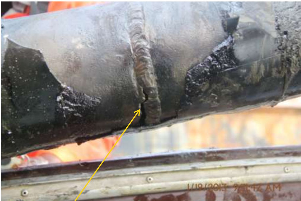
Close up: Failed weld on Kanbo Well5L & S flowline at Amabulu. Picture was taken during Joint Investigation of 19 th January 2013.
