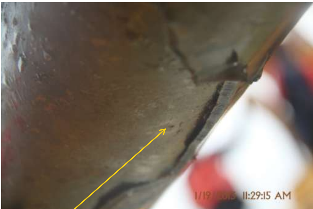
Close up: Pinhole at 6 o'clock position on Kanbo Well5L & S flowline at Amabulu. Picture was taken during Joint Investigation of 19 th January 2013.
