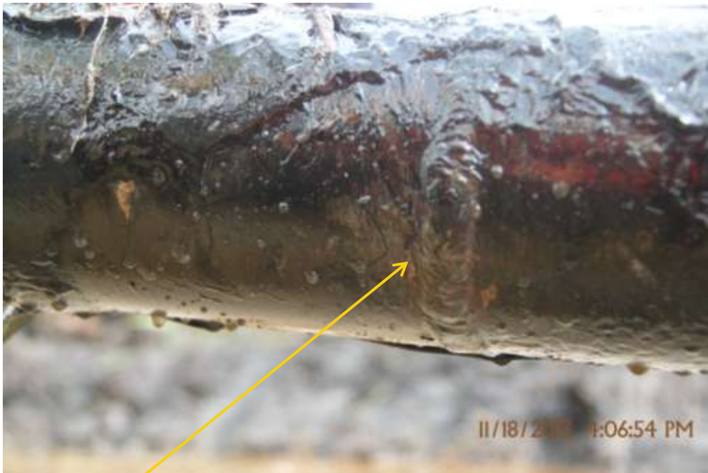
Close up: Failed weld on Kanbo Well5L & S flowline at Amabulu. Picture was taken during Joint Investigation of 19 th January 2013.
