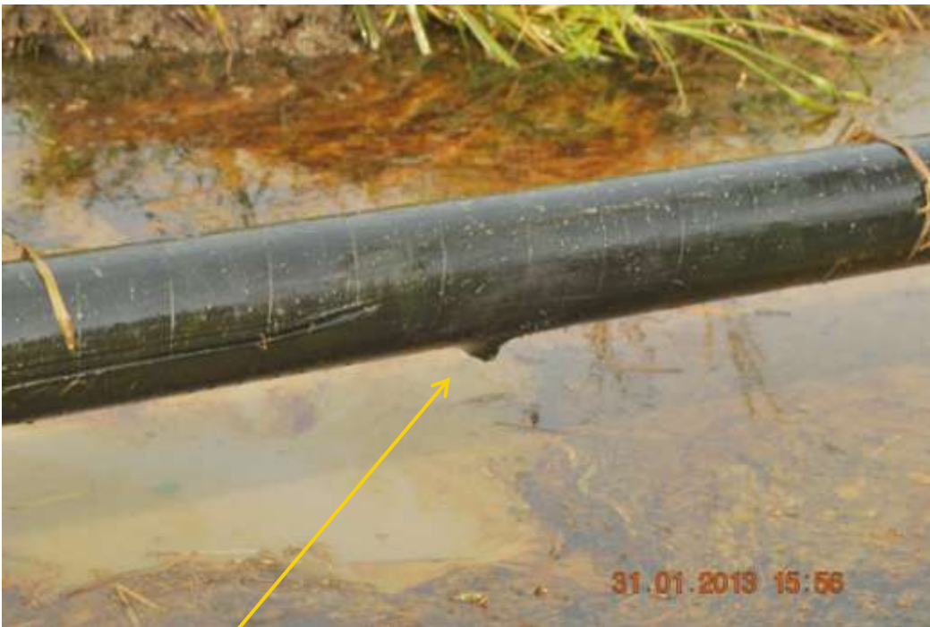
Close up: Bulge due to corrosion on Opukushi Well24T flowline at Agbidiamama. Picture was taken during Joint Investigation of 31 st January 2013.
