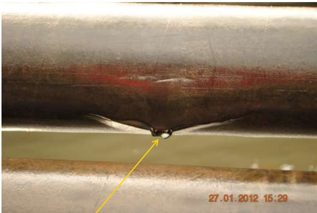
Close-up: Point of internal corrosion on Opukushi Well33L flowline at Egbema-Angalabiri. Picture was taken during Joint Investigation of 27 th January 2012.
