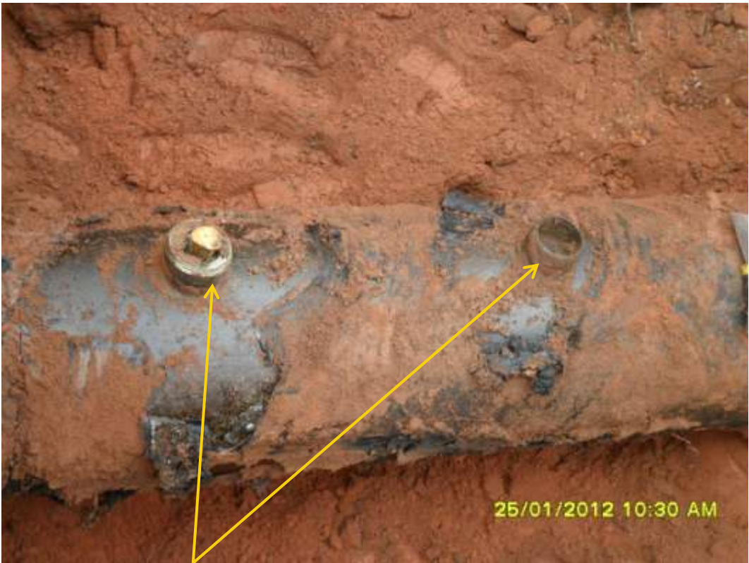
Close-up: Illegal fittings on 16" Egbema-Assa pipeline at Obille. Picture was taken during Joint Investigation of 25 th January 2012.
