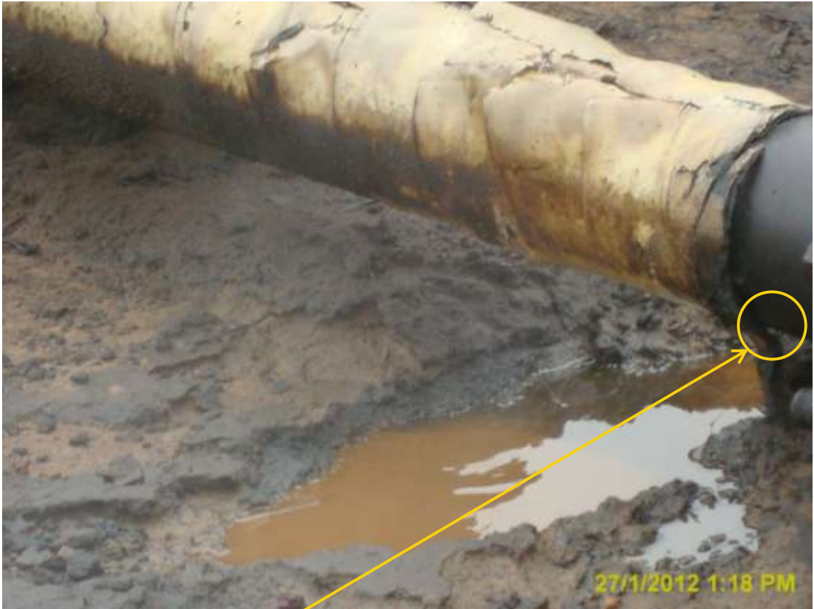
Close-up: Approximate location of hacksaw cut at 6 to 8 o'clock position on Ubie Well9S flowline at Idu/Edrass. Picture was taken during Joint Investigation of 27 th January 2012.
