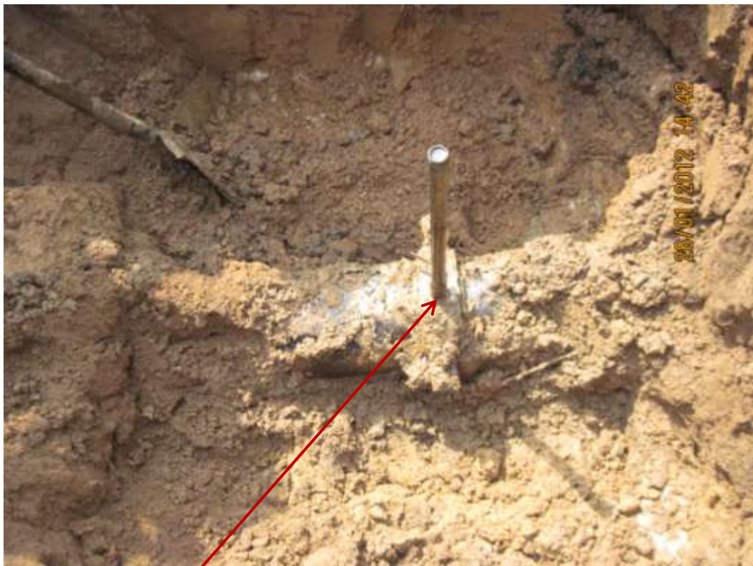
Close-up: Illegal fitting on 8" Umuechem-Nkpoku pipeline at Omunwei, Igwuruta. Picture was taken during Joint Investigation of 26 th January 2012.
