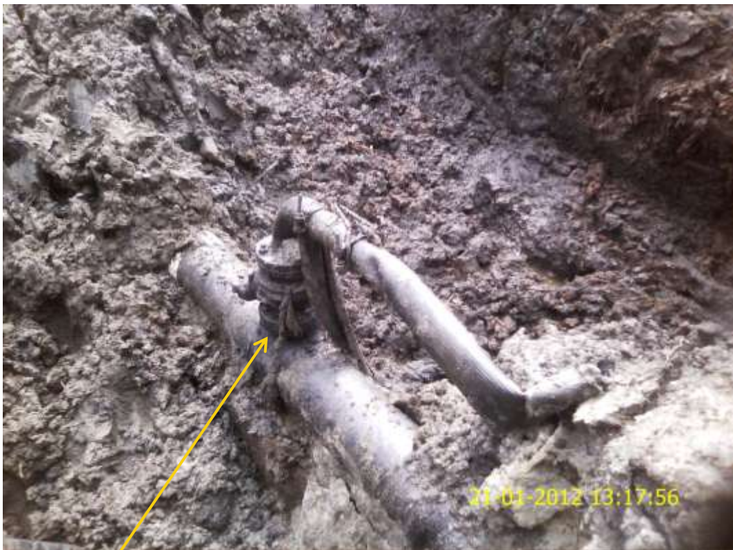
Close-up: Illegal fitting on 8" Cawthorne Channel2 pipeline at Tigerkiri. Picture was taken during Joint Investigation of 21 st January 2012.
