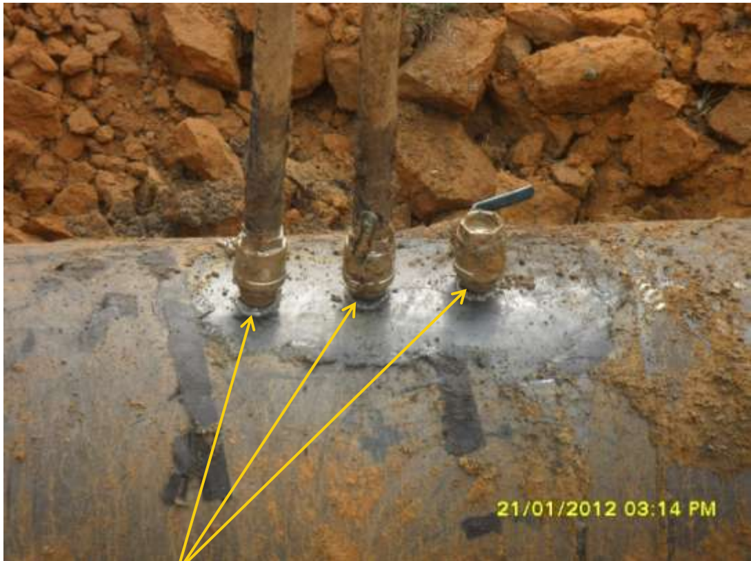
Overview: 2 nd set of Illegal fittings on 36" Npoku-Bomu pipeline at Eneka. Picture was taken during Joint Investigation of 21 st January 2012.
