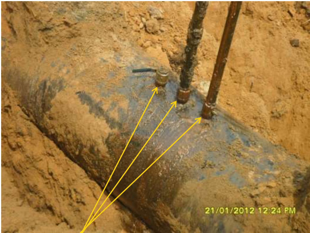
Close-up: 1 st set of Illegal fittings on 36" Npoku-Bomu pipeline at Eneka. Picture was taken during Joint Investigation of 21 st January 2012.
