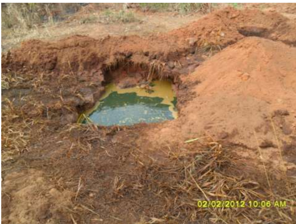
Overview: Part of spill impact on 16" Egbema-Assa pipeline at Assa. Picture was taken during Joint Investigation of 2 nd February 2012.
