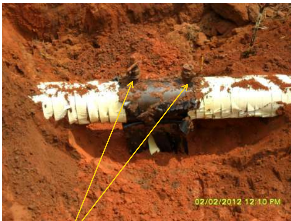
Close-up: Illegal fittings on 16" Egbema-Assa pipeline at Assa. Picture was taken during Joint Investigation of 2 nd February 2012.
