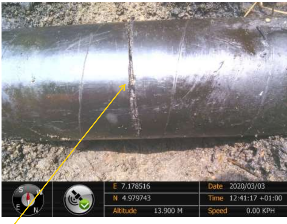
Close-up: Hacksaw cut from 9 -3 o'clock position on 4'' Imo River Well 43T Flowline at Igiriukwu. Picture was taken during Joint Investigation of 3 rd March 2020.
