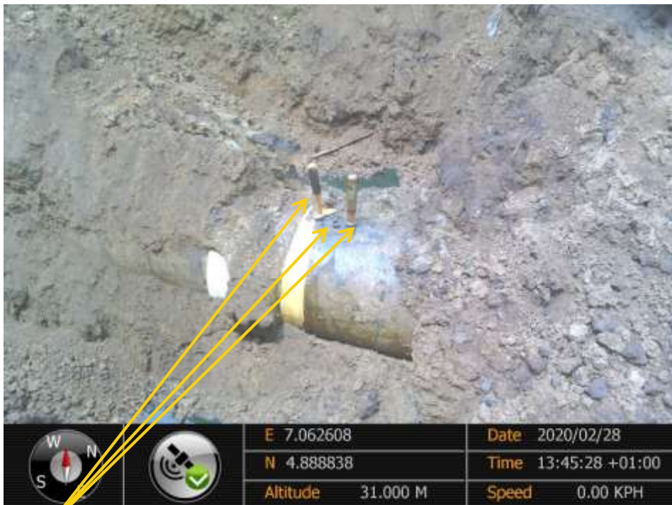
Close-up: 3nos illegal connections( crude theft) installed at 12 o'clock position on 36inch Nkpoku Bomu Pipeline at Atali . Picture was taken during Joint Investigation of 28 th February 2020.
