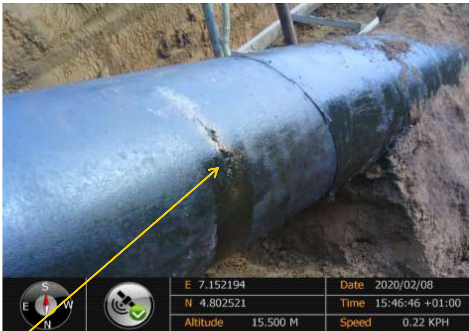
Close-up: Hacksaw cut on 12" Imo River2 – Ebubu Pipeline at Ogale. Picture was taken during Joint Investigation of 8 th February 2020.
