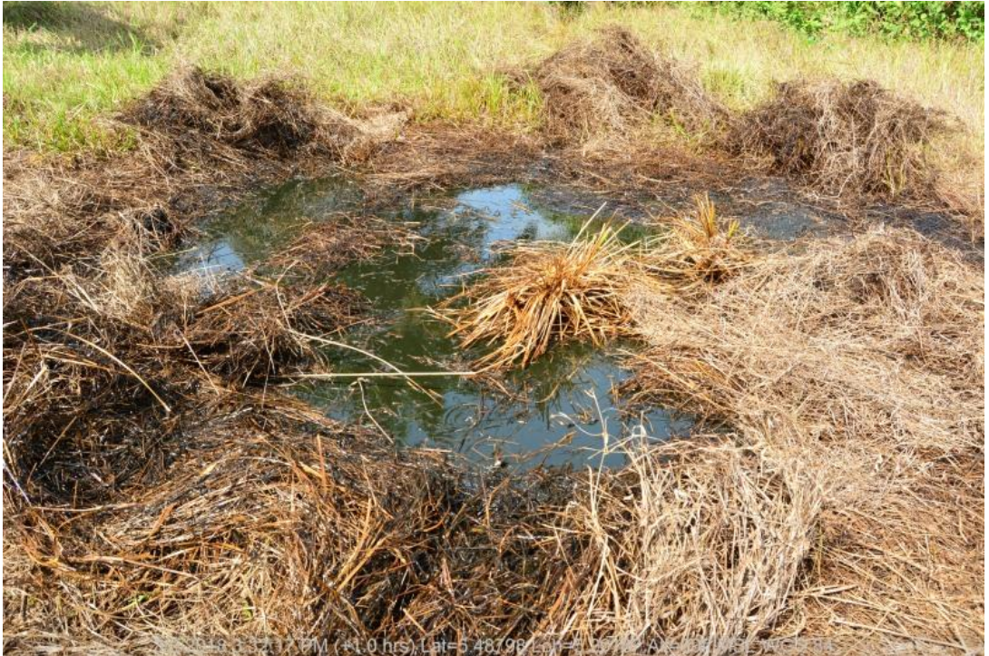
Overview: Part of spill impact on 24" Trans-Escravos Pipeline Right of Way at Sokebolou. Picture was taken during Joint Investigation of 2 nd March 2018.
