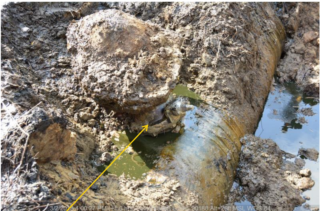
Close-up: Illegal fitting on 24" Trans-Escravos Pipeline at Sokebolou. Picture was taken during Joint Investigation of 2 nd March 2018.
